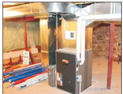
The furnace is busy pumping heat to the Stovewood Building, and heat is being retained by the new insulation, including the insulation sprayed on the stone walls of the basement, which is noticeable to the left of the furnace.
