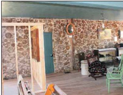
The interior of the store with the construction of the "new post office" on the left
