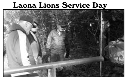
The Laona Lions worked together with the Forest County ATV club and Wabeno Lions to spruce up the trail. The Group got together on Saturday October 22nd to install a gate on the trail, brushed and did repairs.
