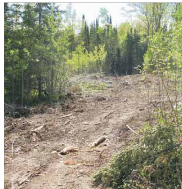
This is a new wooded trail under construction that will lead the rider through a wooded setting with everything from rocks to mud to navigate with his 4x4.
