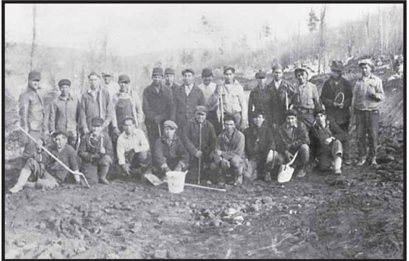
We take our roads for granted, and when it is a road that has served the area for many decades, we have no idea of the labor it took to build the road. This old picture is from the Colburn collection, and is likely from the Wabeno area. Who needs a dozer or a dump truck when you have lots of labor?
