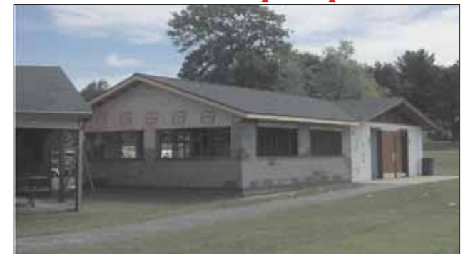
The new pavilion was being worked on last Tuesday to get it ready for the big Summerfest event this Saturday. As can be seen, it is connected to the beach house and will have a working kitchen with hot and cold water, sink and all the amenities. The old structure on the left will remain as a pavilion.
