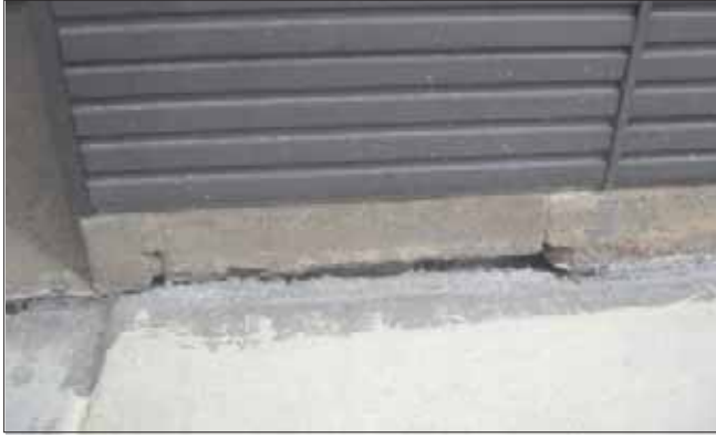
Cracks between the building and the sidewalk, that weren't there before the latest sidewalk project are numerous around the downtown. Crandon Pharmacy is the site of this crack, and they have many more.
