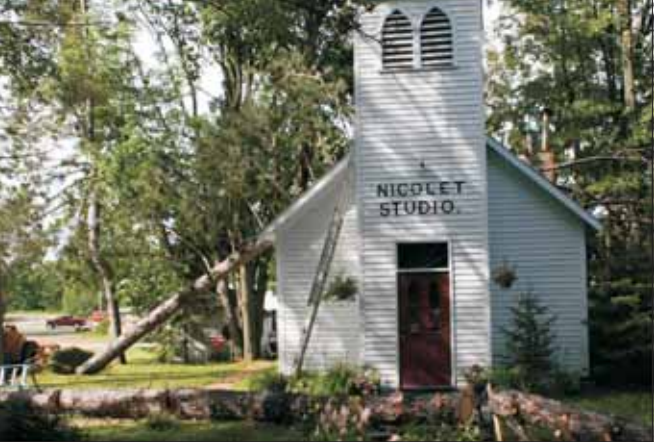
Joan White's studio in Lakewood was decorated with a big red pine across the roof. Fortunately, it didn't appear that there was major structural damage to this unique business place.
