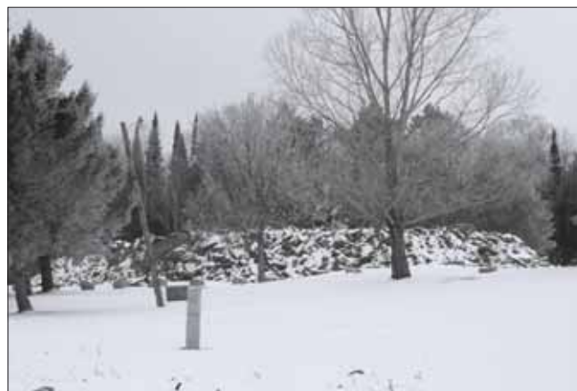
The photo on top shows the fill dirt that is raising the level of the park to prevent problems with wet campsites. The road is the old level of the ground.
