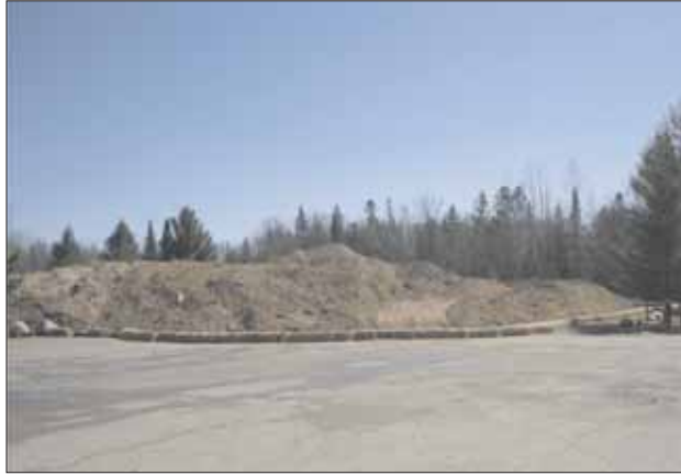
This massive pile of fill dirt is in the parking lot at the Veteran's Memorial Park. There is a pile of top soil in the middle of the fill dirt to finish off the project. It will be spread when the ground dries out enough to hold up the equipment.
